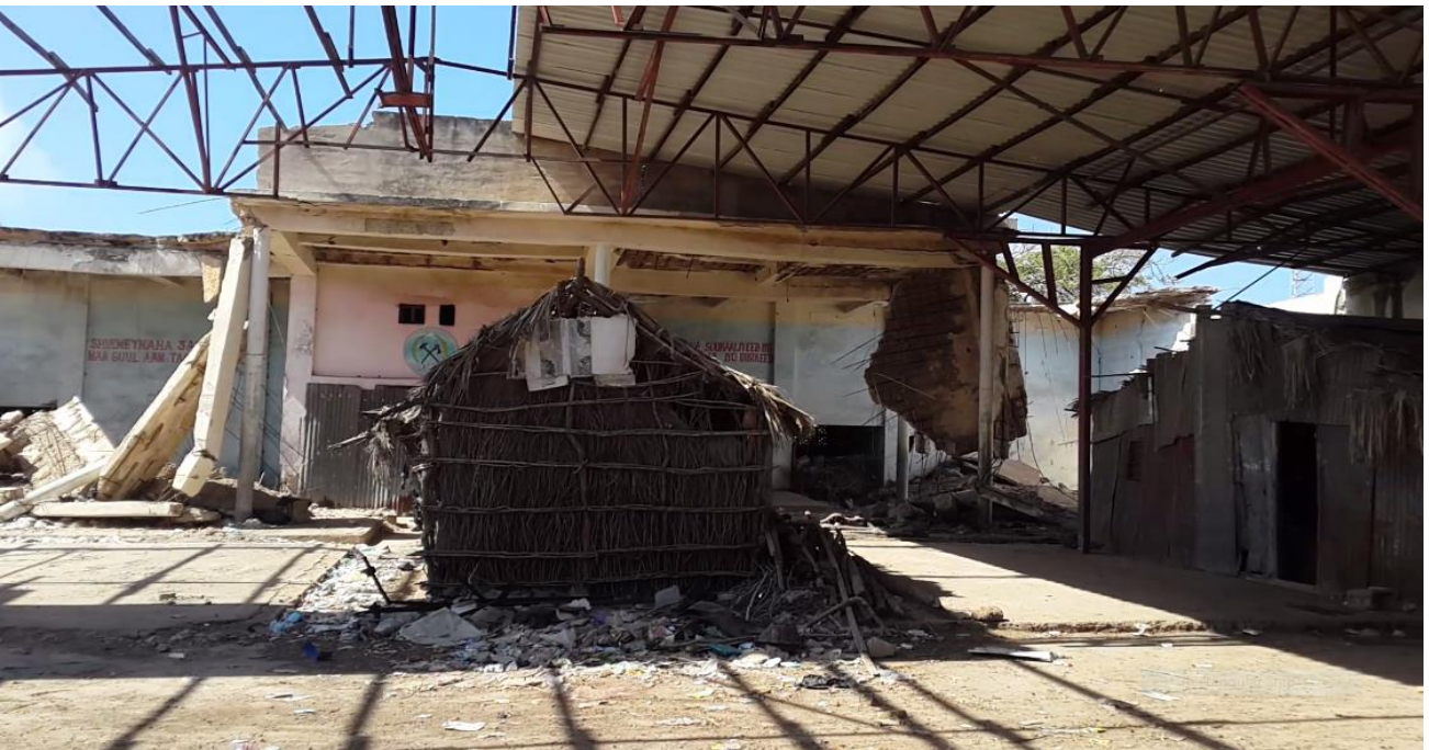
Photo 4: Inside and Entrance of the Old Kismayo theatre during engineering measurement exercise
